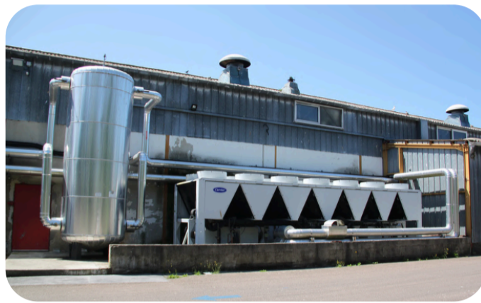
Heat recovery system
