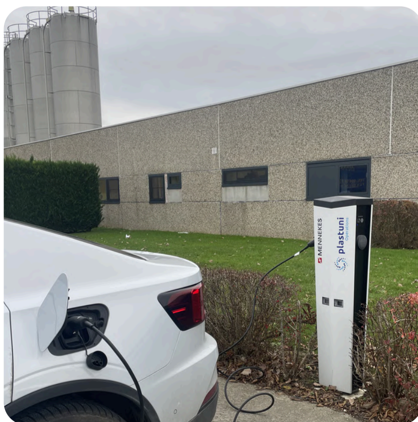
Electric vehicle charging stations - Plastuni Operations
