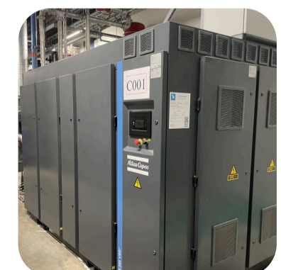
New compressor - ANL Wellen
